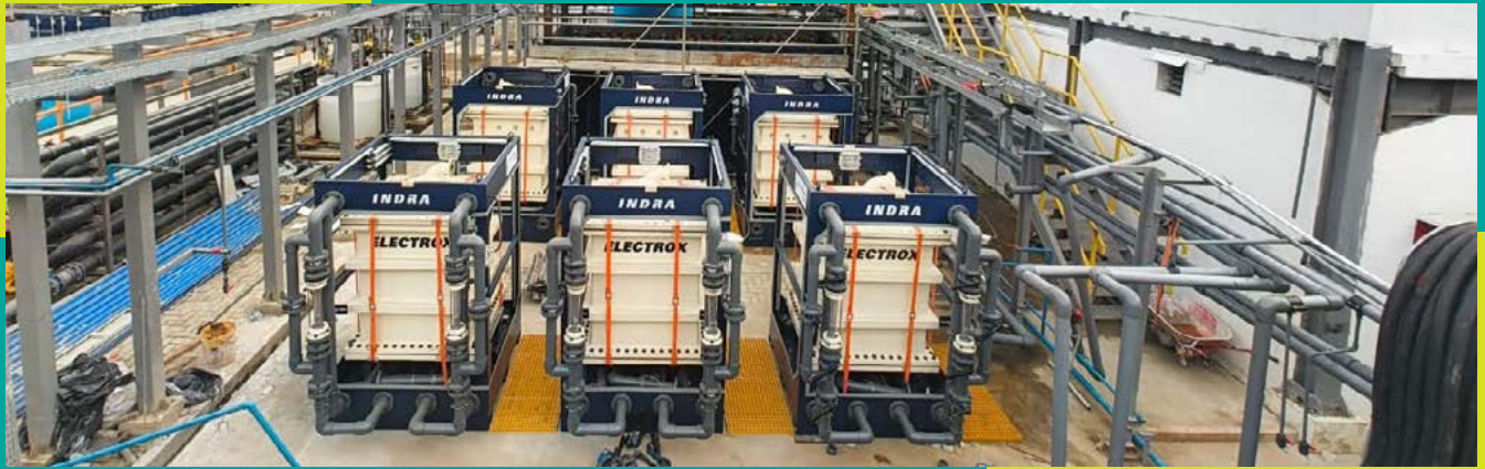
✓ Indra Electrox Modules installed at a FMCG facility producing soaps, hygiene & personal care products in Medan, Indonesia, to treat oleochemicals wastewater (1650 m 3 /day)
