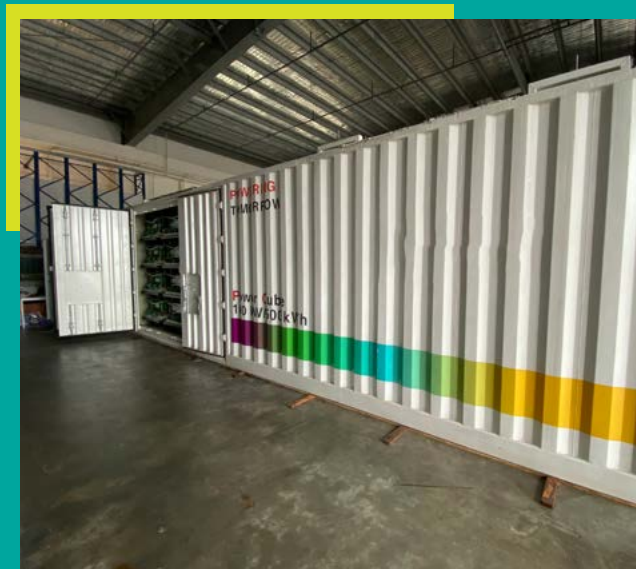
VFlowTech's 500kWh battery
