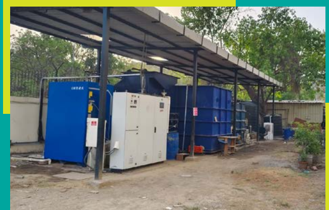
✓ Indra Electrox Module installed at a textile facility in Noida, India, to treat garment washing and coloured wastewater (66 m 3 /day) for process reuse
