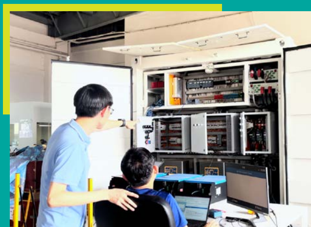
VFlowTech's Singapore Team members carrying out software testing and battery integration
