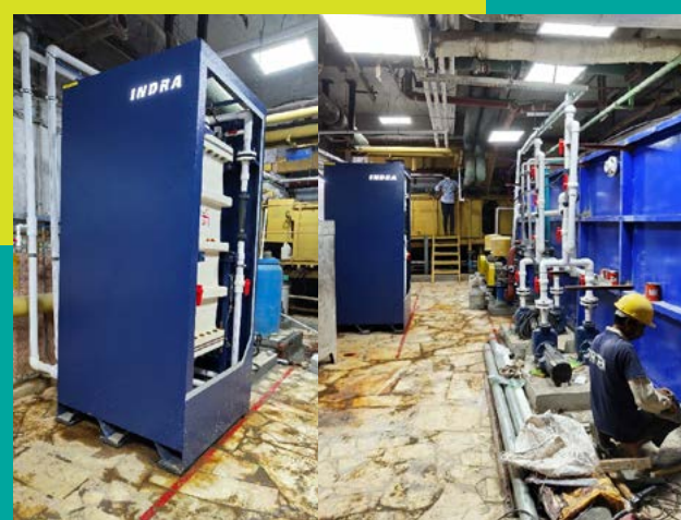
✓ Indra ElectroX Modules installed at a hotel in Mumbai, India, to treat laundry effluent (80 m 3 /day) and sewage (blackwater & greywater - 250 m 3 /day) for water recycling and non-potable reuse
