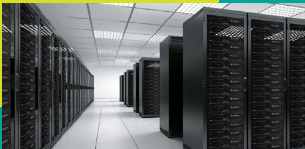
A typical data centre facility
